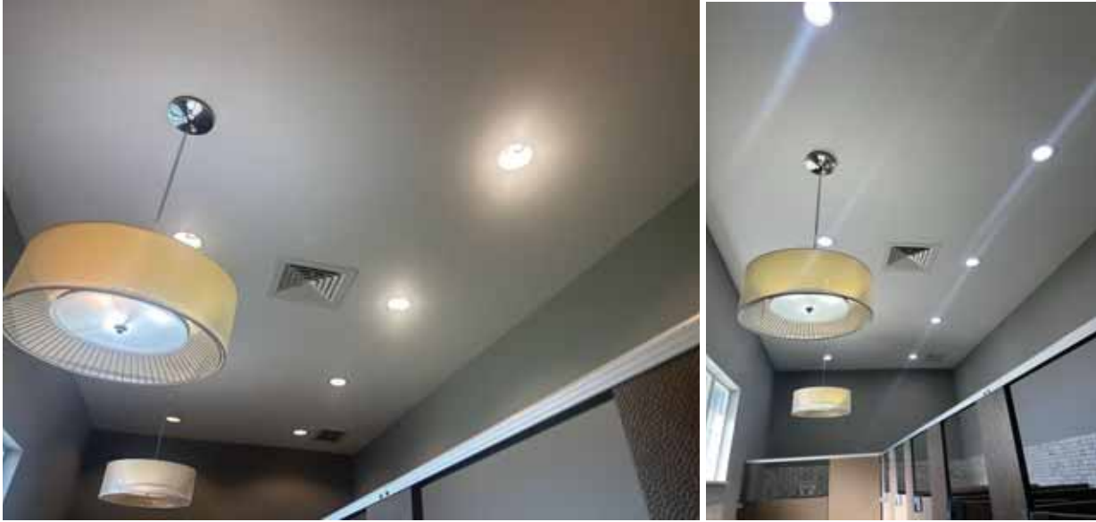
Hallway Lighting Before and After
