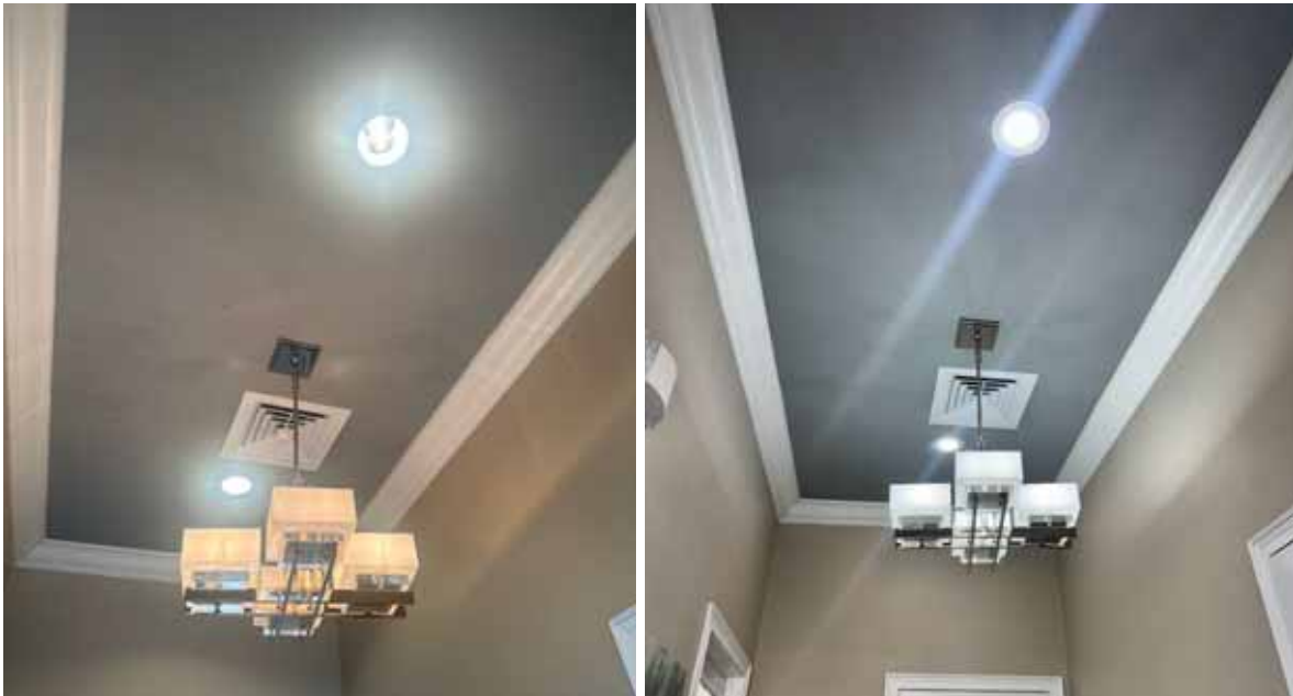
Hallway Lighting Before and After
